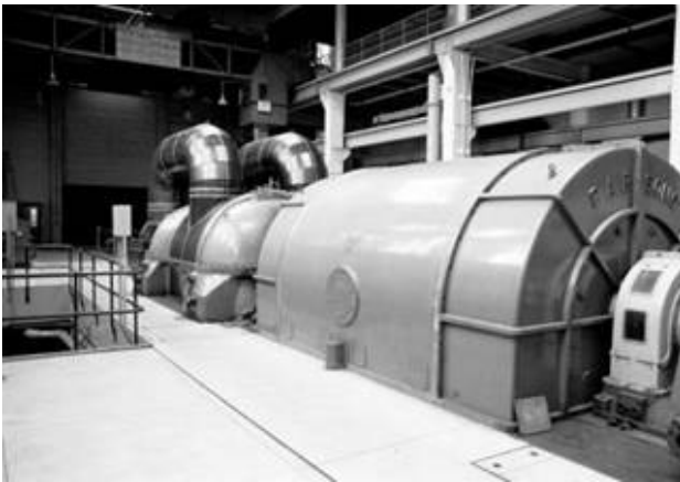
East Yelland Steam Turbine
